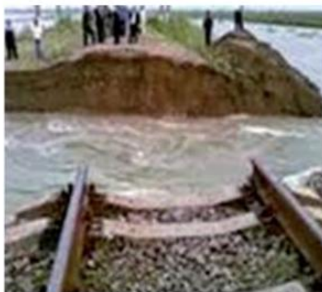
Fig. 5.3: Damage on railways caused by flooding of the Kura River in Azerbaijan, with maximum water level from 18–21 May 2010. Source: National Hydrometeorological department of Azerbaijan
