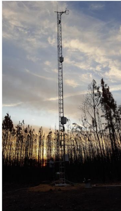
Fig. 1: The 12m slim tower with the eddy-covariance system immediately after its installation (photograph: J. Jacob Keizer, 22 September 2017).
