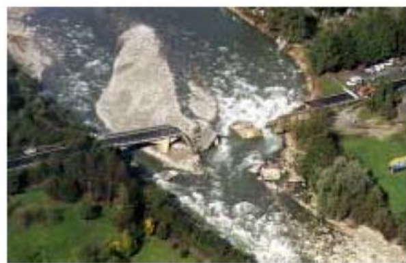
Fig. 2 Aerial view of the collapsed bridge 'Ponte Sul Sangone', Giaveno, Province Turin (Italy) from October 2000 (Picture: http://www.provincia.torino.it/emergenza/ )
