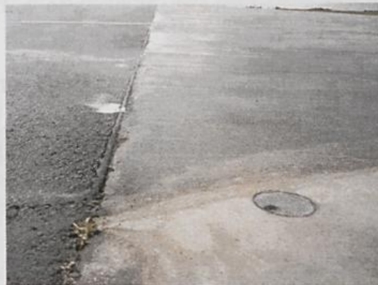
Figure 6: Water film sensor and the surrounding paved area. The sensor has dried-up even though the paved area is still moist.
