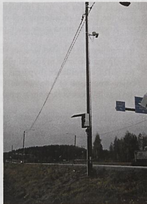
Picture 4. Camera at site (device cabinet opened)
