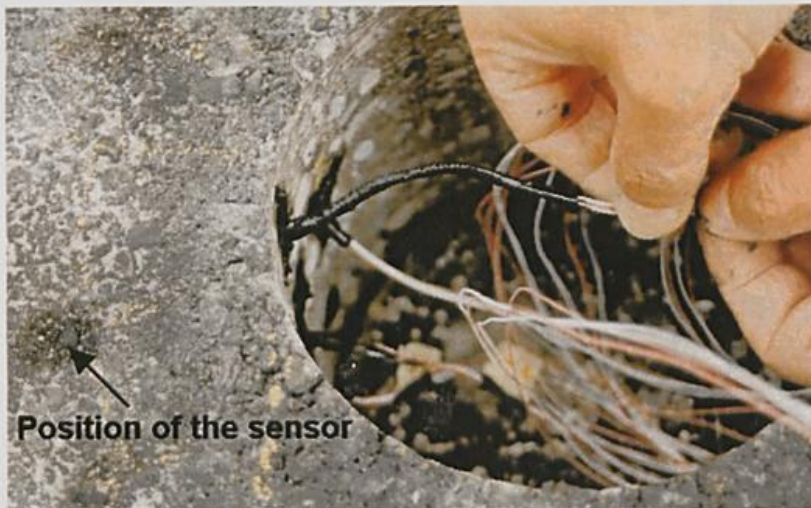
Figure 2: Installation of a sensor for roadway surface temperature on the roadway surface
